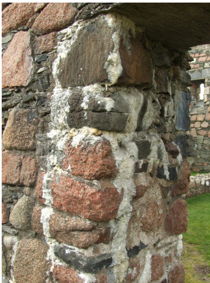
Figure 3 : Washing out of wall core mortar resulting from water penetration to open wall heads, typical of many unroofed ruins. Higher rainfall levels are likely to increase such problems (Image: Historic Scotland).
